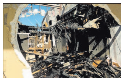
Eli Segall Las Vegas Review-Journal The abandoned building at 5285 Dean Martin Drive shows extensive damage on Thursday after a two-alarm fire.
